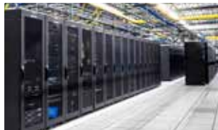
Data server room
