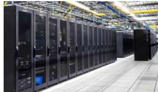
Data server room
